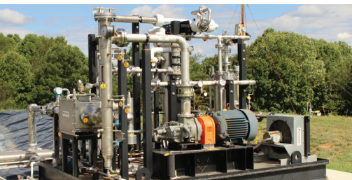
Lloyd Ray Farms | Swine Waste to Energy Project, Yadkinville, NC
