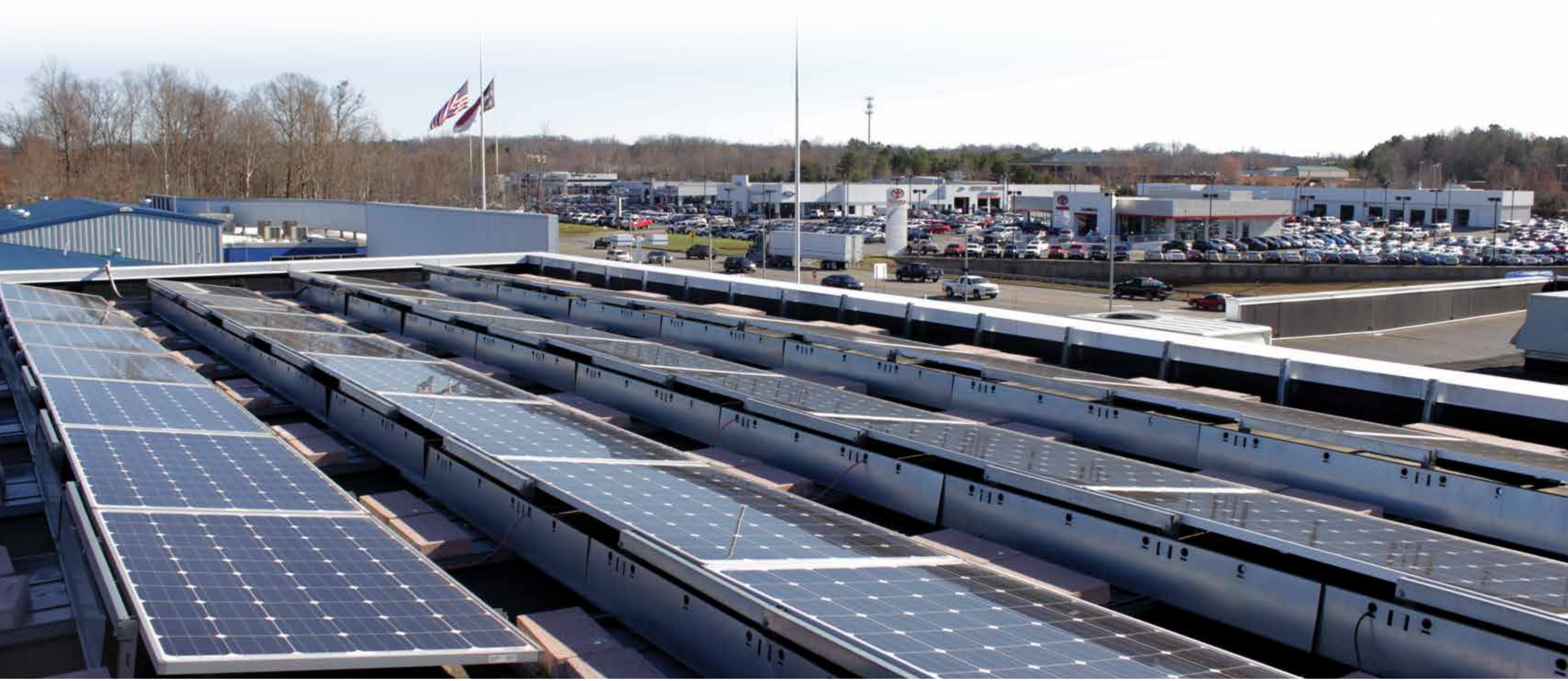
Solar Project at Gerry Wood Chrysler Dodge Jeep Ram in Salisbury, NC
